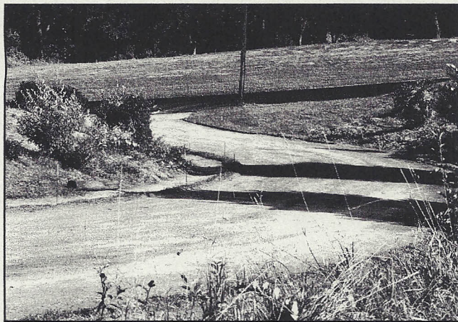
Preparation work for paving the driveway at the Coley house coordinated by Joe Spetly.
