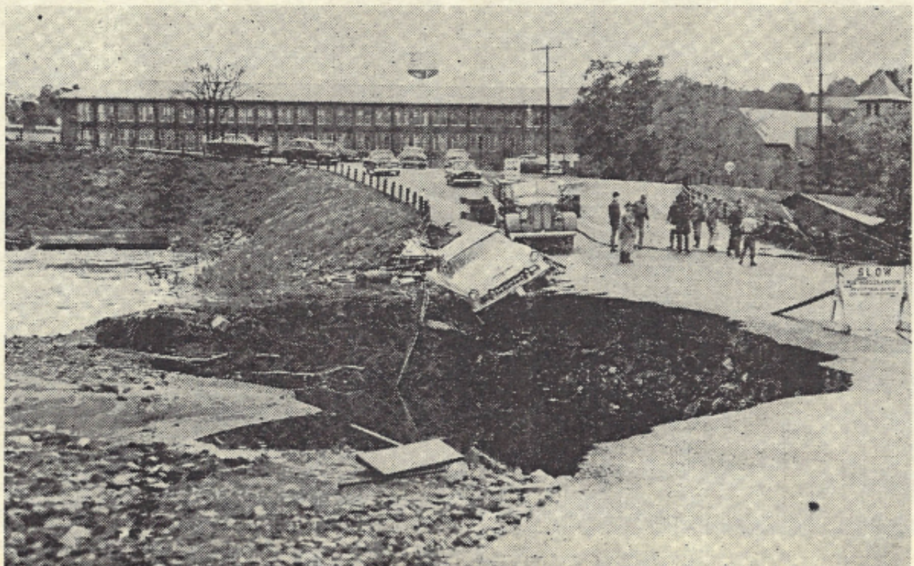
An automobile came to a perilous stop on the edge of this gaping hole in the new Georgetown Overpass approach, and its five occupants were rescued 90 minutes later. When Clarence Korker took this picture Sunday afternoon a crowd was gathering to see what could be done to get the car off its perch. Holes like this one, some bigger, some smaller were common sights throughout this area.
